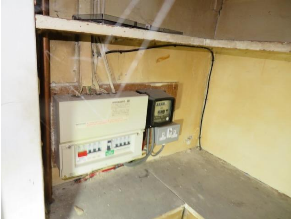
Photo 14 – Electrical meter and consumer unit.
