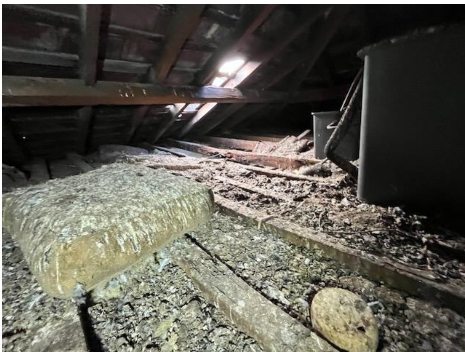
Photo 11- Guano covered timbers above collapsed first floor ceiling
