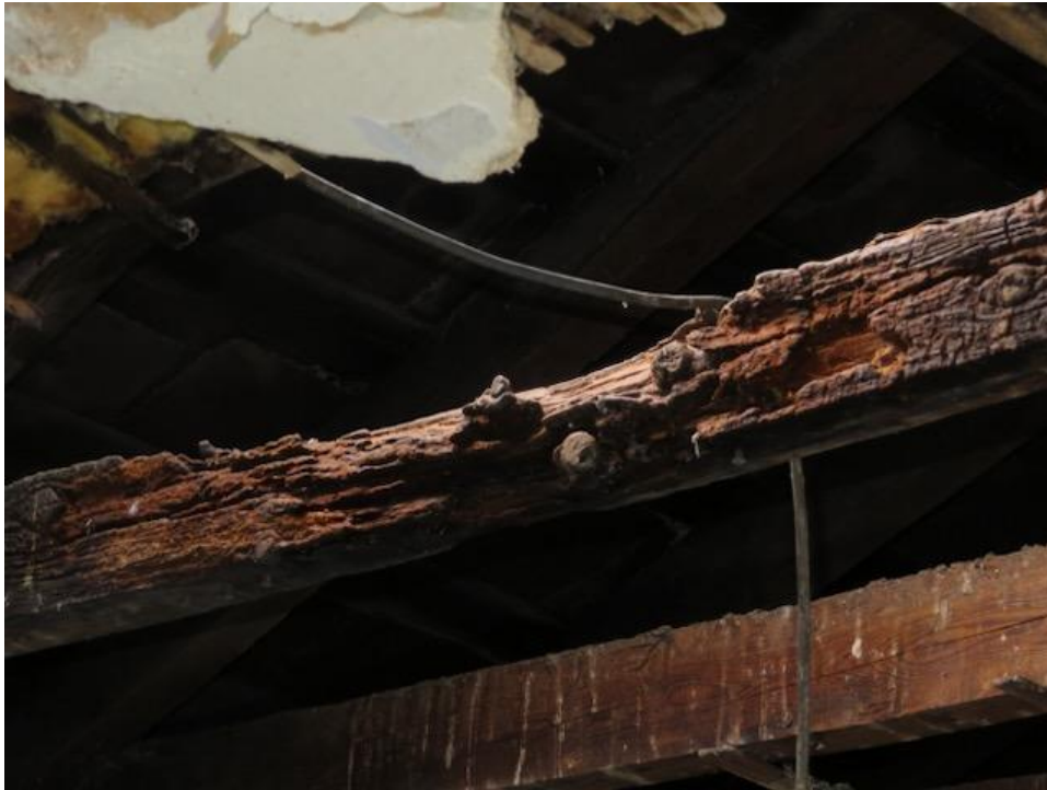
Photo 8- Rotted through roof tie
