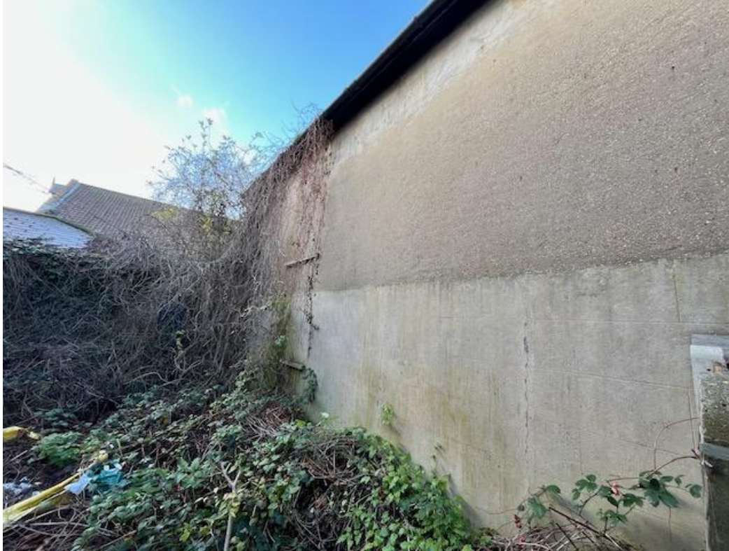
Photo 3 - Cracked render overgrown with shrubs
