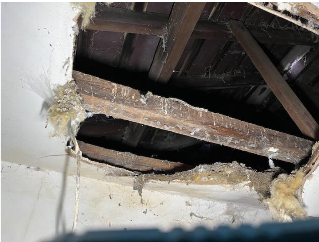
Photo 7- Guano covered timbers above collapsed first floor ceiling
