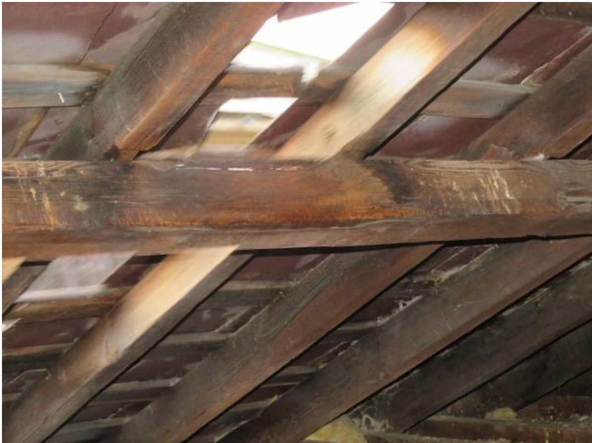
Photo 4- Holed Roof timber structure
