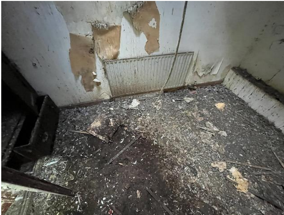
Photo 10- Guano covered first floor finishes
